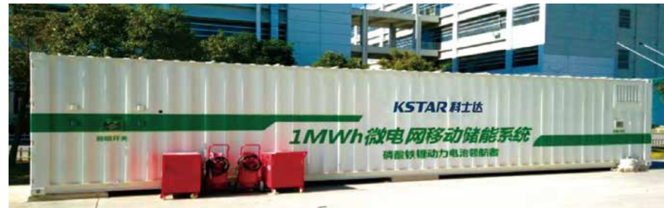
► 3MW/12MWh BESS Demonstration Project in Shenzhen
