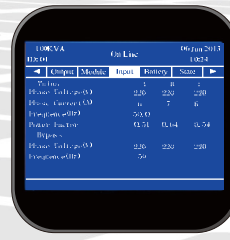
UPS Cabinet Control Panel
