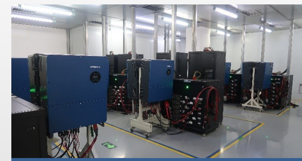
Inverter Ageing Test System
