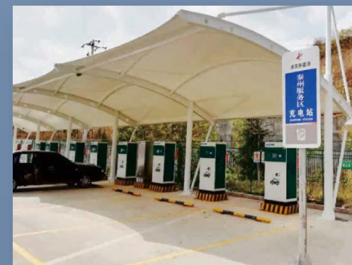
Qinzhou Expressway Service Area
