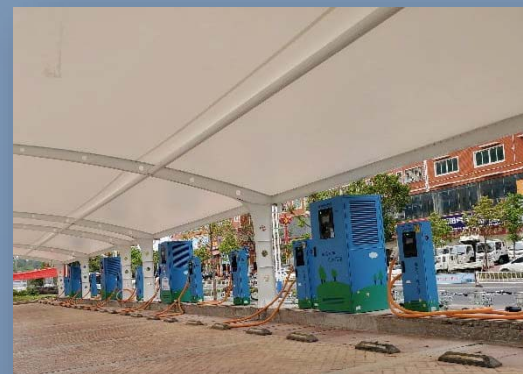
Fujian Investment Public Charging Pile
