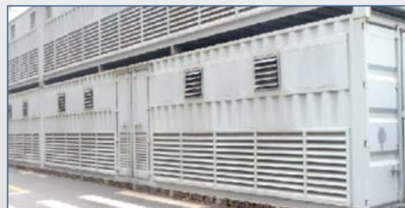
Load Test (2MW)
