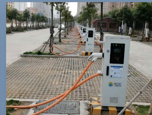
Ningde Communications Investment Public Charging Station
