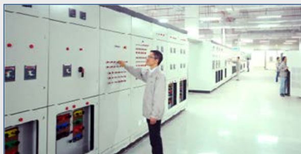
R&D Test (2MW)
